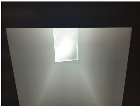
Paint overspray 1st Floor skylight
