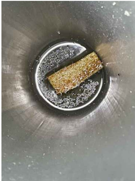
Bath. Timber inside drain
