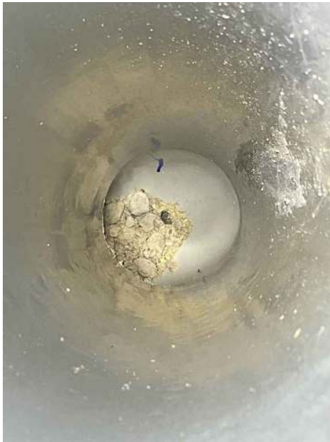
Laundry. Gravel inside drain
