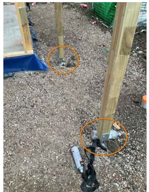
Porch posts no barrier installed
