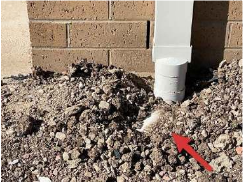
stormwater pipes must be the required depth below the future concrete paving. weep hole clearance allowed for. Rear
