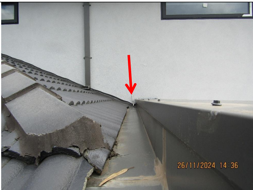
Photograph 22. shows the area where water ingress has occurred into the roof cavity, over the laundry. Note the 100mm depth required for a box-gutter at the end and wall junction has not been achieved. The building contractor has put lead flashing at the wall and valley gutter junction only.
