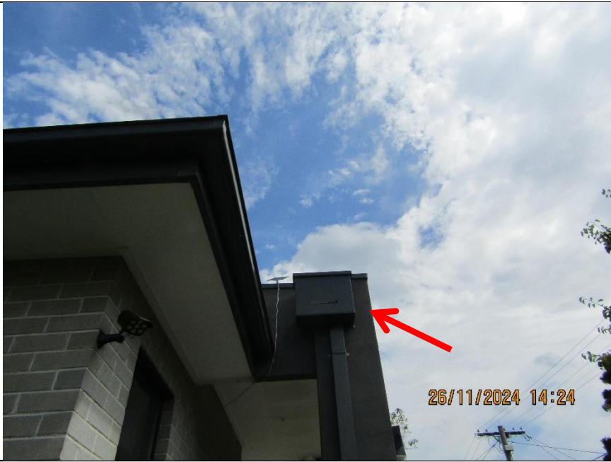
Photograph 15. shows the front porch and rain-head including overflow slot which is not compliant. The rain-head is not dispersing rain water to the atmosphere during a heavy rain event adequately due to poor installation.
