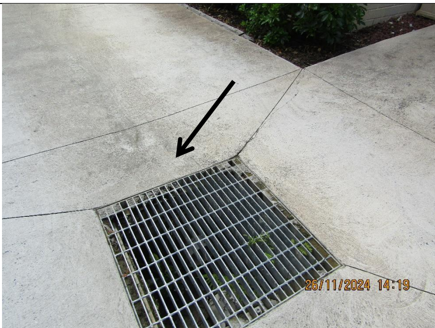
Photograph 12. shows the civil drainage storm water system and a compliant pit 4 with a 150mm drainage sub-surface pipe. This pit and staining debris around the pit indicate overflowing during heavy rain events.
