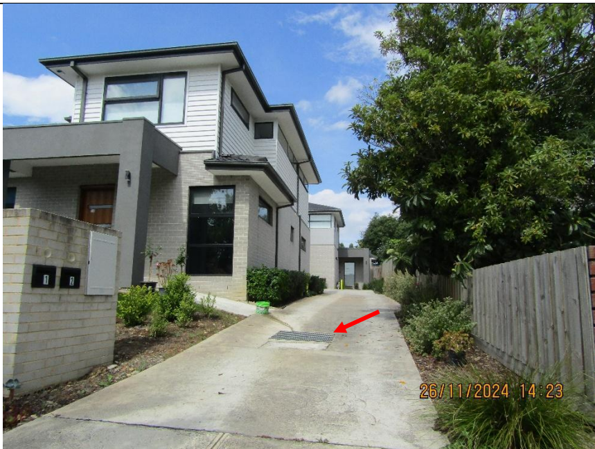
Photograph 10. shows the front drive way and civil pit 5 as being observed as non-compliant and not approved as civil drainage design by the local council Civil Division.
