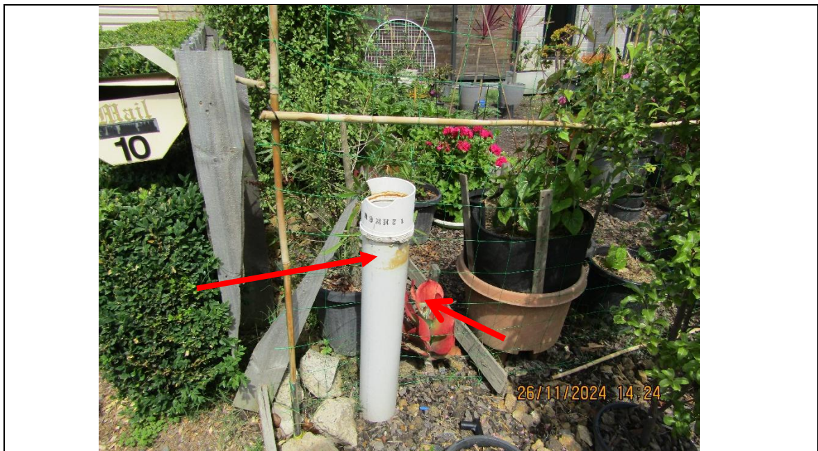
Photograph 8. shows the front section of the residence and the storm water point which required a storm water pit 4 not installed. This is considered in-complete building works by the building contractor.
