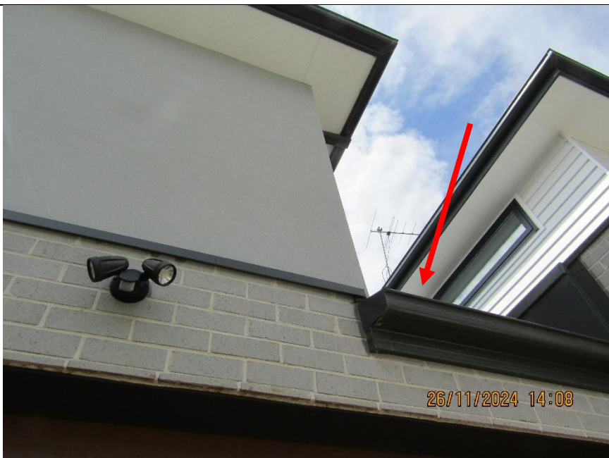
Photograph 4. shows the garage overflowing gutter during heavy rain events. No water ingress damage was observed to the garage. Water overflowing to the gutter and down pipe was evident.
