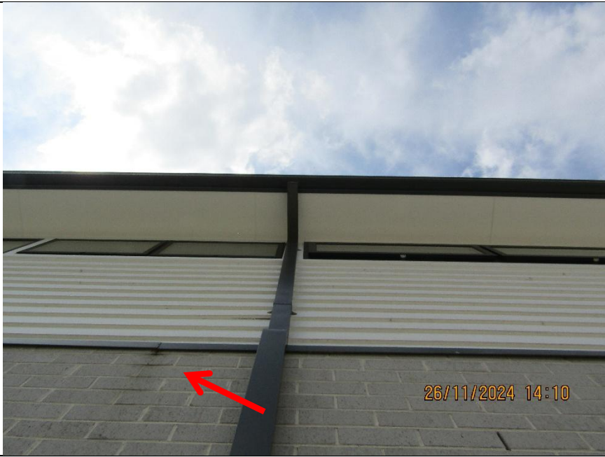
Photograph 5. shows the external southern elevation and water staining from a wall flashing. The wall flashing has not been correctly installed.
