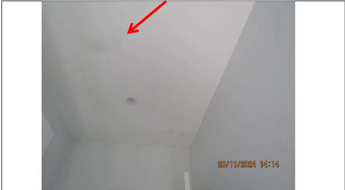
Photograph 7. shows the internal laundry painted plasterboard ceiling with water stains and mould due to long term water ingress from a failed roof drainage system.
