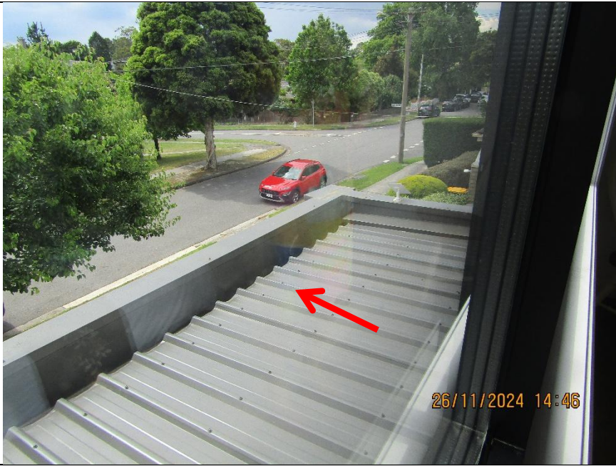
Photograph 17. shows the front porch and roof cover which is designed only to accommodate for a small roof surface area of storm water drainage.
