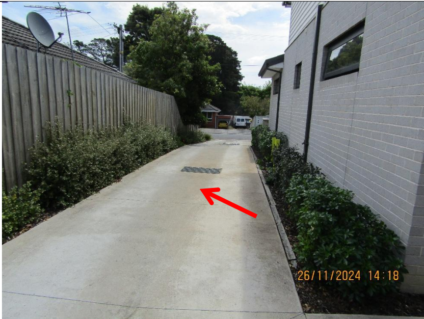
Photograph 11. shows the civil storm water drainage system and pit 4 which overflows during heavy rain events.
