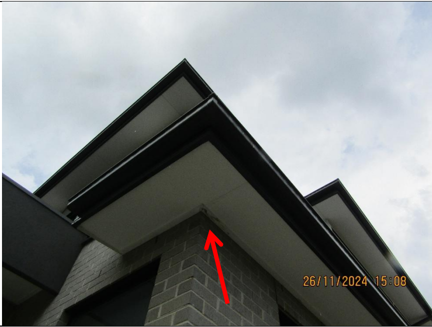
Photograph 3. shows the side south elevation and damaged eave lining from water ingress from overflowing gutters. This is due to blockage and restriction of the storm water system.
