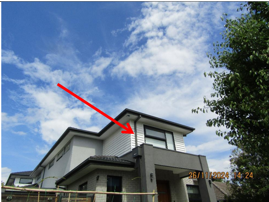
Photograph 18. shows the upper roof and roof drainage down pipe dispersing additional storm water onto the porch roof cover. This is non-compliant building work as the porch was not designed to take the rain water from the upper roof. This also contravenes the hydraulic design of the roof.
