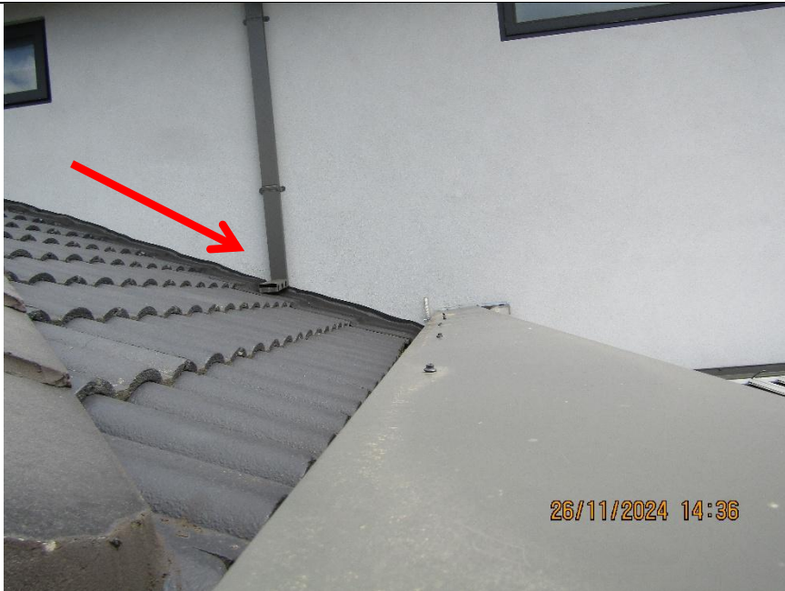
Photograph 21. shows the spreader downpipe dispensing large amounts of water into the valley gutter. The valley gutter cannot cope with heavy rain events and subsequently water is entering the roof cavity over the laundry.
