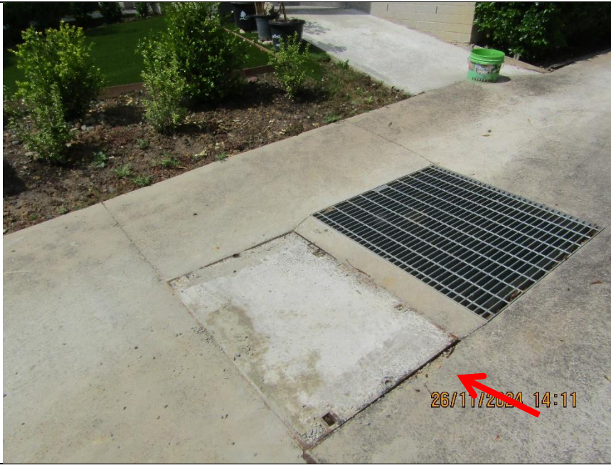
Photograph 9. shows the front civil storm water drainage system and Pit 5 which has not be certified by the local council Civil Engineer.
