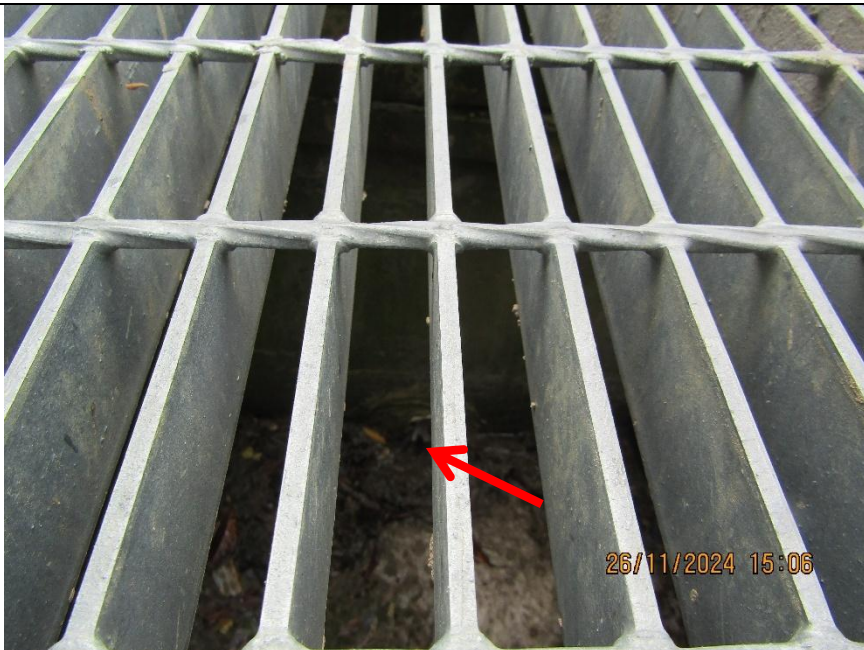
Photograph 14. shows the civil drainage pit 5 and a crushed and compromised storm water pipe within the pit. This is contributing to a poor flowing storm water drainage system during heavy rain events.
