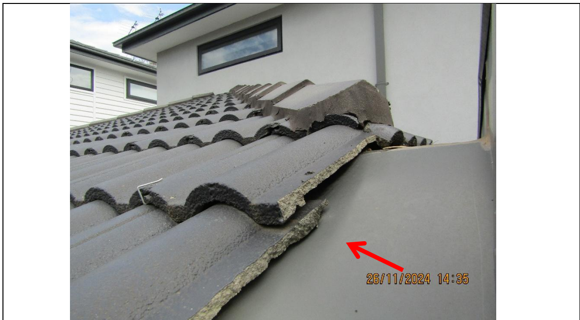
Photograph 20. shows the non-compliant valley gutter in lieu of a required box gutter. This valley gutter cannot cope with heavy rain event allowing water ingress within the roof cavity.
