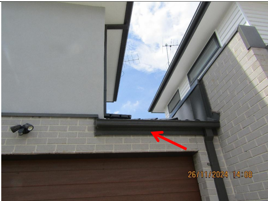
Photograph 6. shows the side garage section where water ingress has been alleged to have occurred. No visible water ingress damage was observed. Evidence of water marks does indicate a blocked or non-functioning roof drainage gutter and down pipe.
