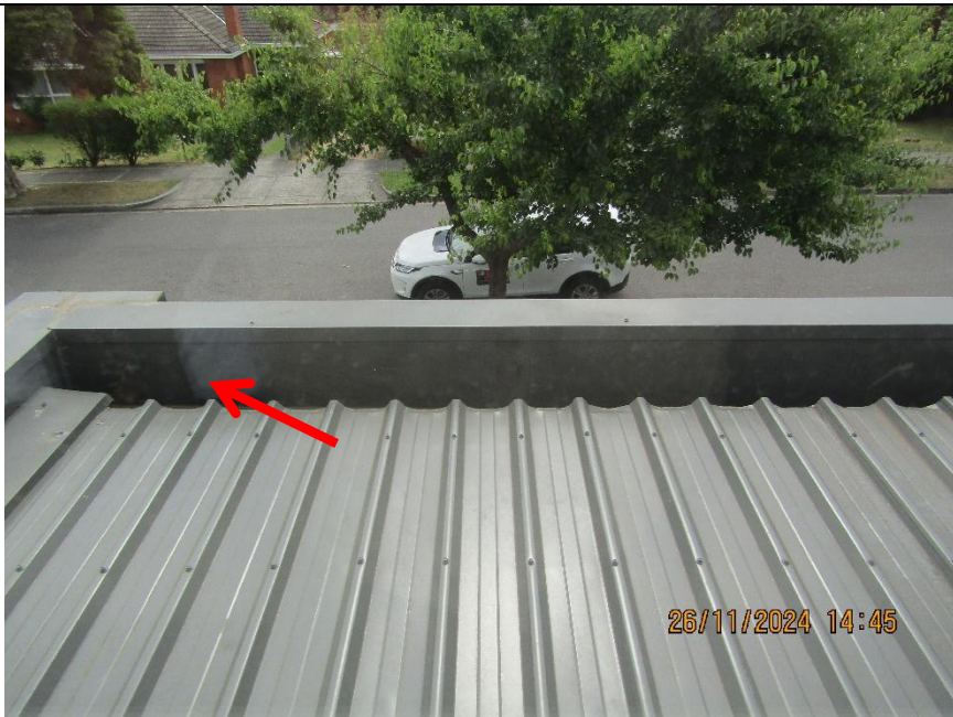
Photograph 16. shows the box gutter which is filling and overflowing into the porch roof cavity during heavy rain events.
