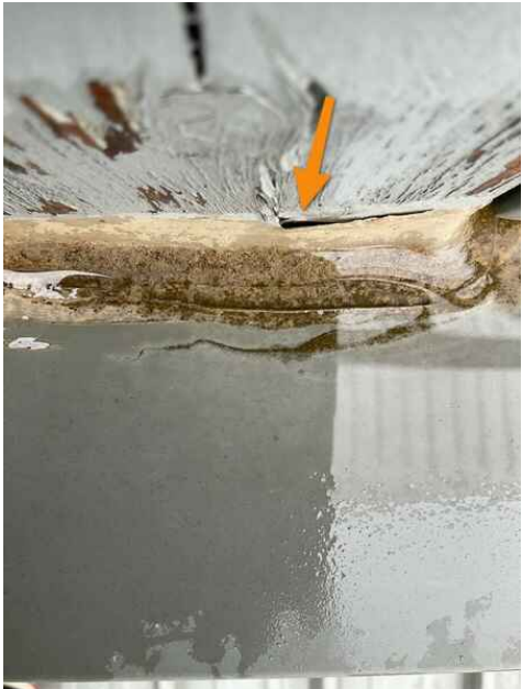
Silicone has degraded and a hole is present
