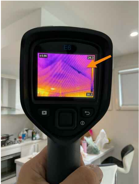
Moisture evidence after hose test to timber post
