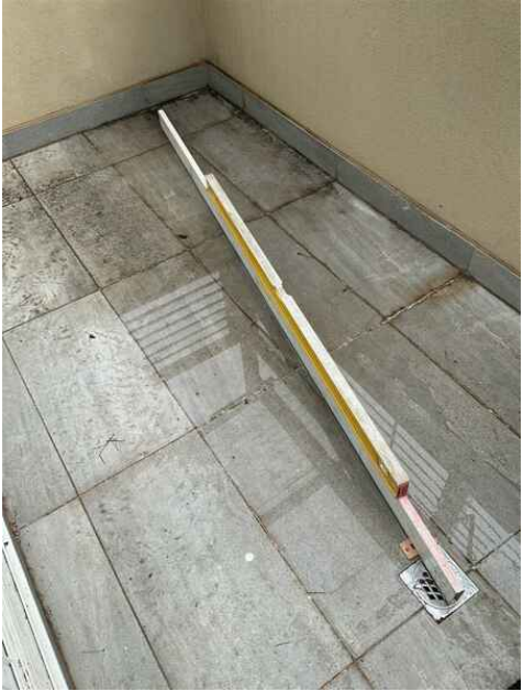
5mm fall over 2m - Insufficient
