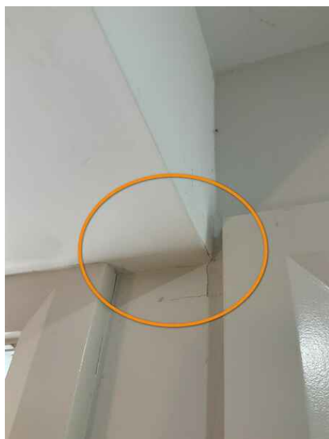
Plaster cracking due to water ingress
