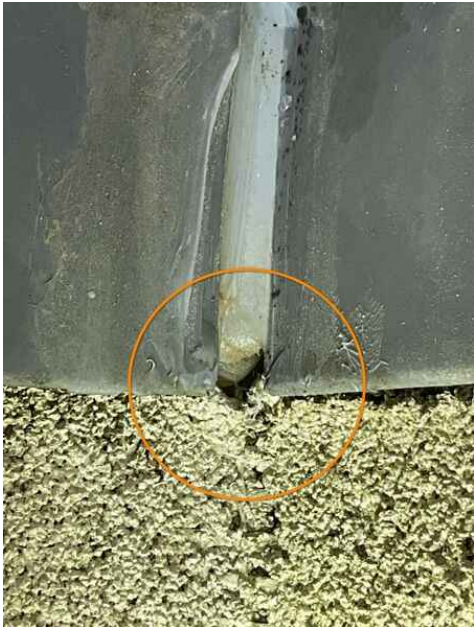
Hole in flashing at corner of balcony
