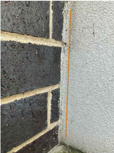
Render crack to be repaired watertight
