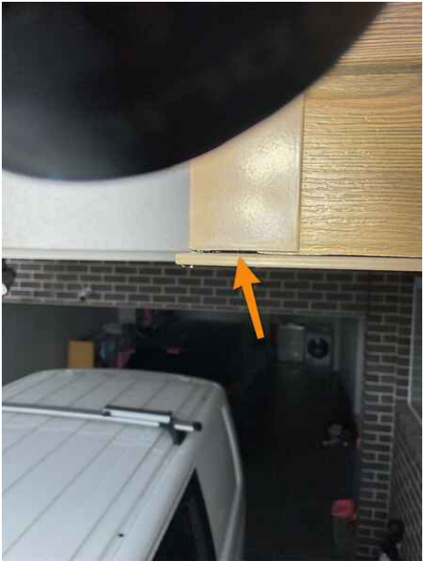
Euroclad Vertical Started Profile is not falling away from the ceiling. It is falling towards the ceiling
