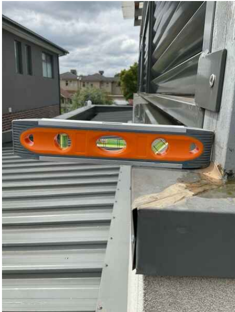
Negative fall towards timber posts which is causing water to pond around the timber post
