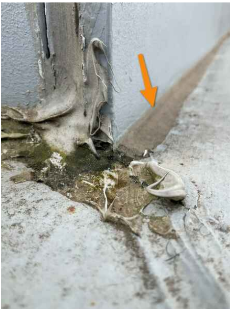
No 6mm gap and silicone installed between sill flashing and matrix cladding.
