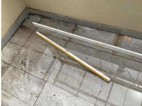
Negative fall where ponding begins
