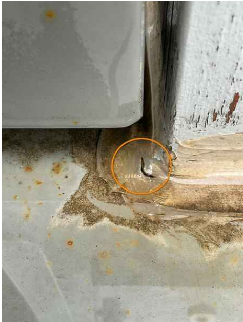
Hole to silicone at timber post to metal flashing connection
