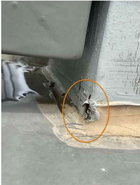
Sealant degraded to Timber post to metal capping connection.
