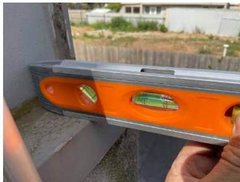
Negative fall to sill flashing.
