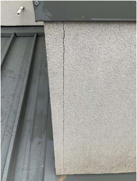
Render crack in this area above water stain
