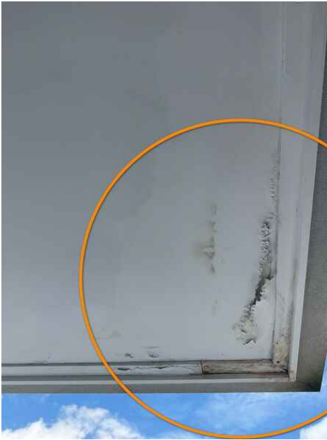
Visible water damage
