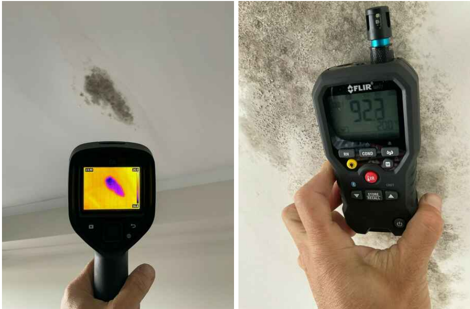
Moisture reading after hose test. Reading shows high moisture reading
