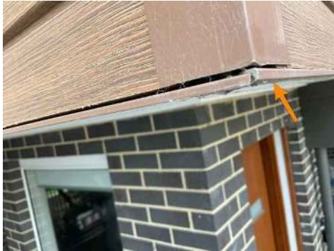
Left side of flashing has the required fall, the right side does not
