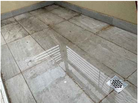
Water ponding to balcony
