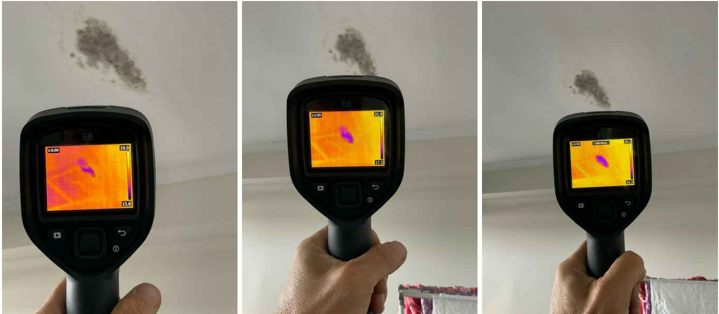
Moisture increase with time, as water ponds to the balcony.
