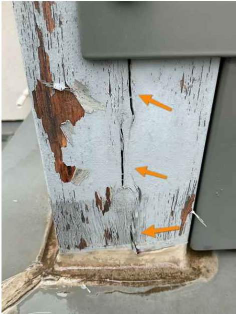
Cracks in timber post which can allow water ingress to travel past the timber post to metal flashing connection
