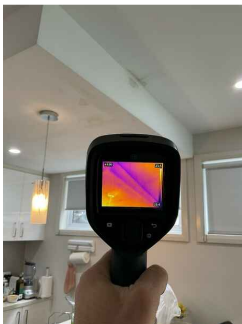
No moisture prior to hose test
