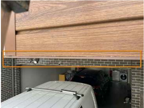
No gap left to bottom to drain water away.
