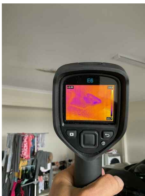
Additional leak towards the front of the garage.
