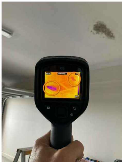
2 x locations to garage showing water ingress
