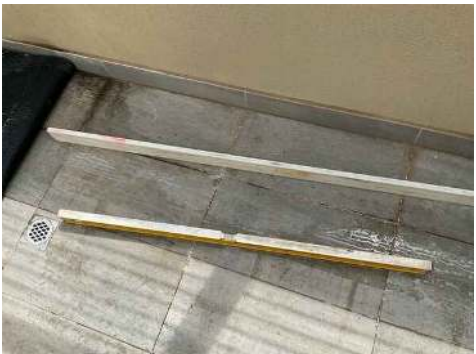
Floor is level for the first 1200mm away from the drain.
