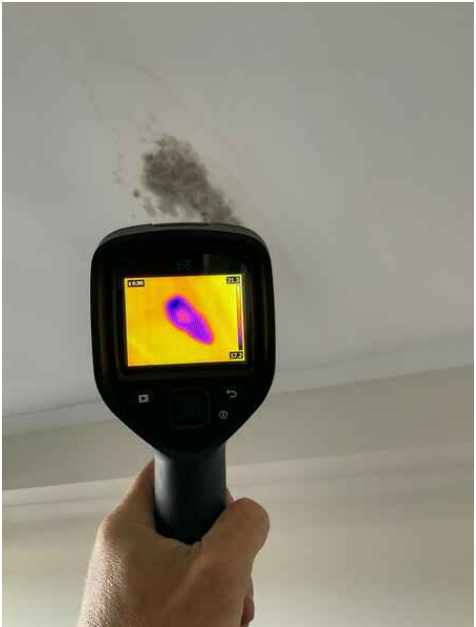
Hot water spray test at timber post to metal flashing connection, and the hole to render underneath flashing at corner of balcony
