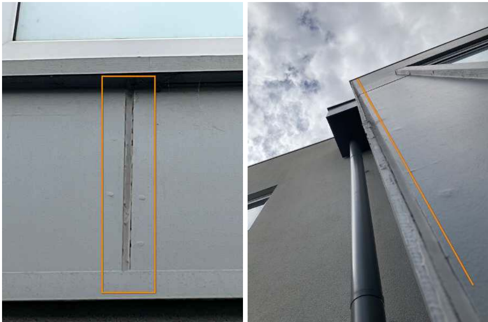
Matrix to be fully resealed to front facade
