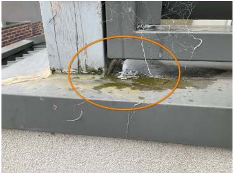
Water ponding adjacent to post connection
