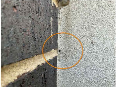
Holes to cladding
