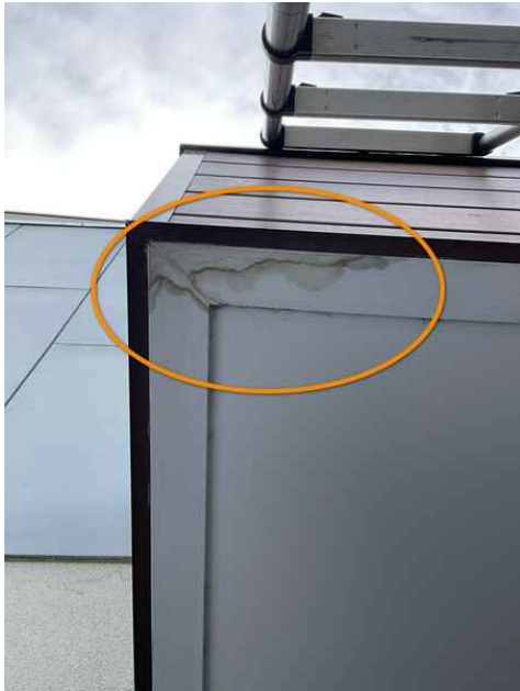
Visible water damage
