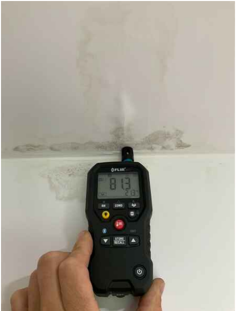
High Moisture reading after hose test
