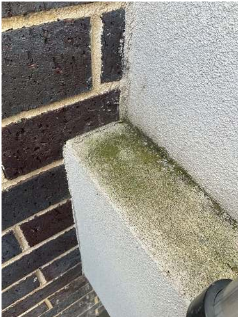
Ponding water. No flashing installed
