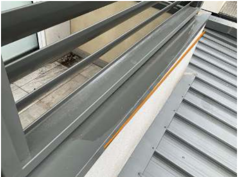
Water ponding to cappings adjacent to post
