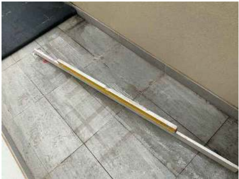
3mm fall over 2m - Insufficient
