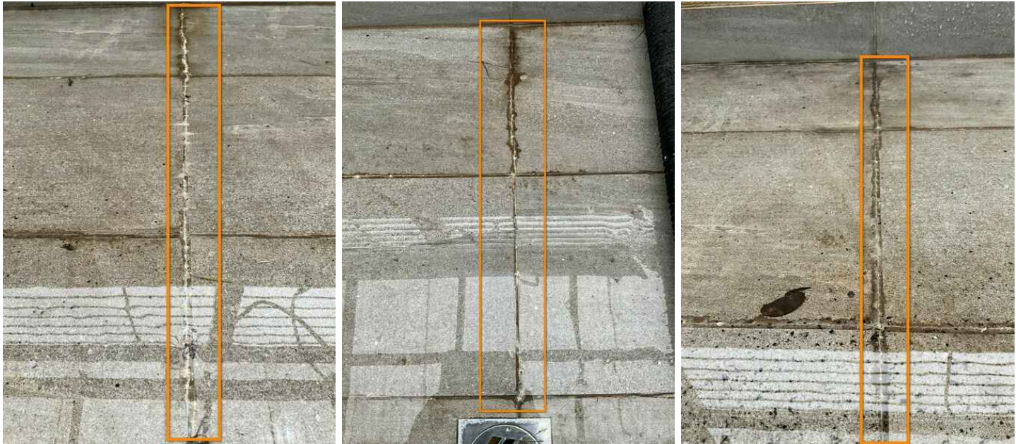
Efflorescence to balcony tiles below ponding water
