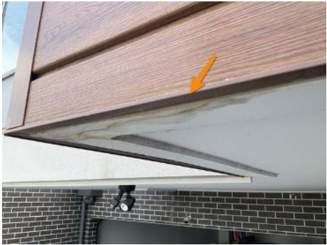
MDF used for external trim, is swollen due to moisture and needs replacing.
