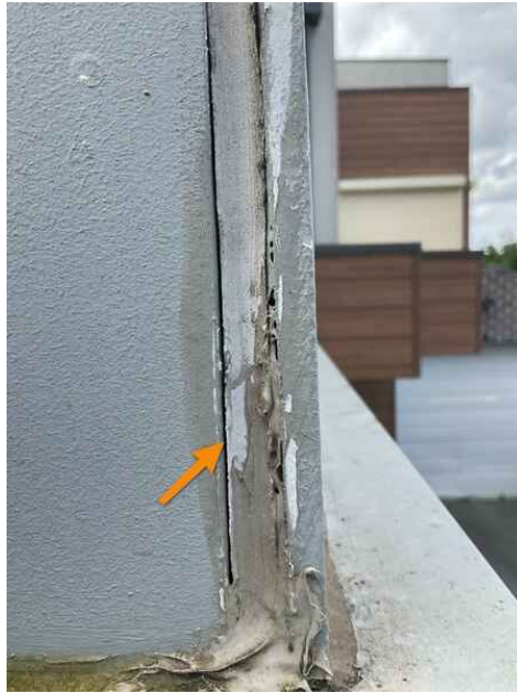
Matrix cladding joints require re sealing. - Homeowners Maintenance
