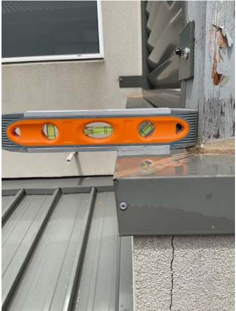
Negative fall towards post to flashing connection
