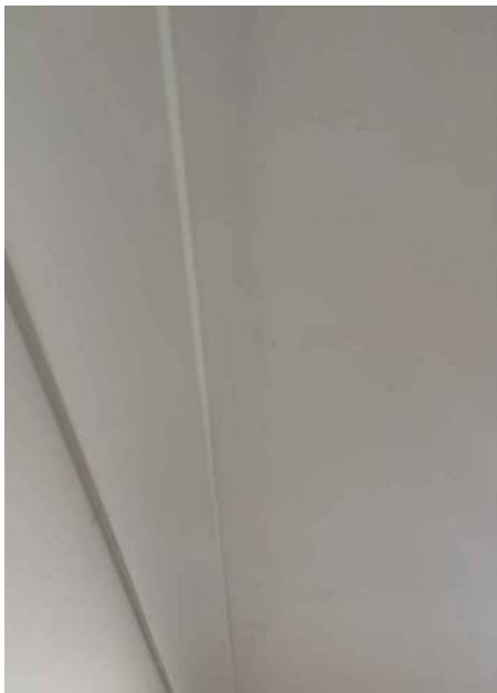
evidence of staining into the Cornice ceiling junction
