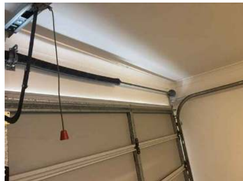
Garage opening head and door opener viewed from within the garage — head / lintel zone (Item 3 garage lintel reported unmarked and corroded).
