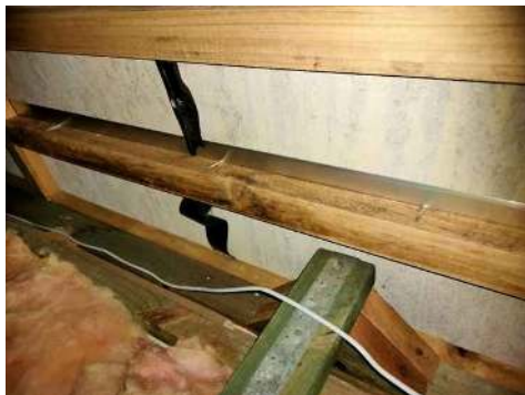
Roof-space view of the external wall build-up behind the cladding — timber framing, sarking and services visible; Fixings missing supporting battens.
