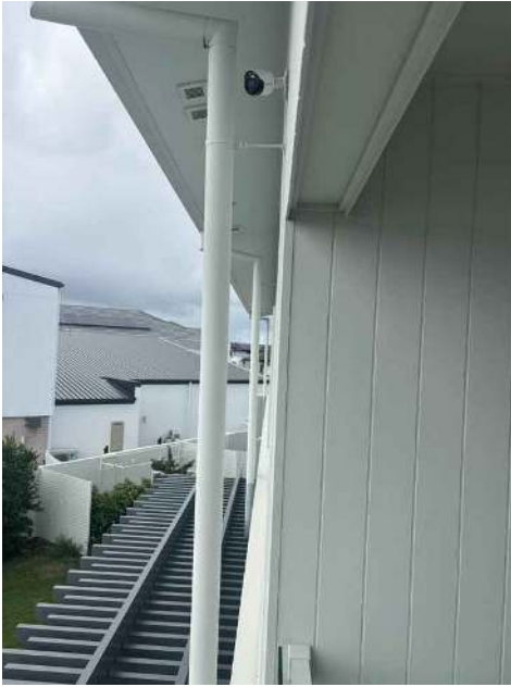
Downpipe at the eave / fascia corner running down past the Axon cladding — upper bracket fixing location to be assessed for corrosion (Items 19–20).
