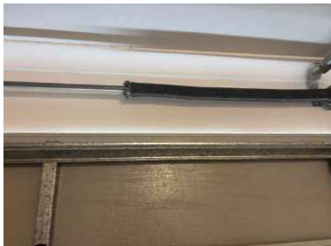
Garage opening head viewed from within the garage — sectional door head and track at the lintel zone (Item 3 garage lintel reported unmarked and corroded).
