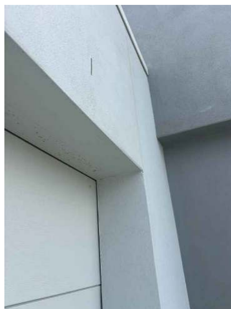
Rust spots forming on the lintel above the garage. - this side faces away from the saltwater canal.
