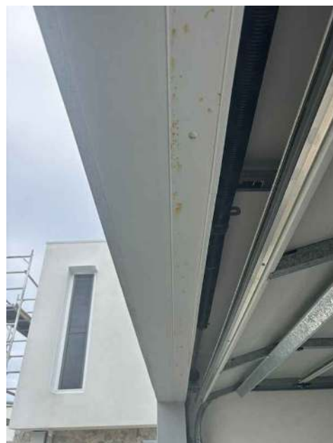
Eave / balcony soffit underside with rust-coloured staining and cladding above, scaffold and neighbouring dwelling beyond — coastal exposure and roof-edge detailing.
