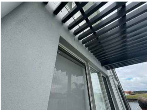
Axon-clad wall with a downpipe — context for the downpipe bracket corrosion assessment (Items 19-20).
