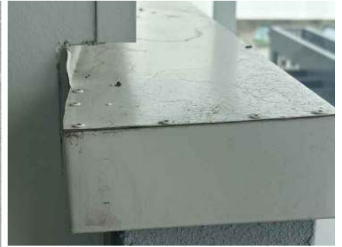
Upper flashing between 1st and ground floors - has been laid with a fall INTO the property.
