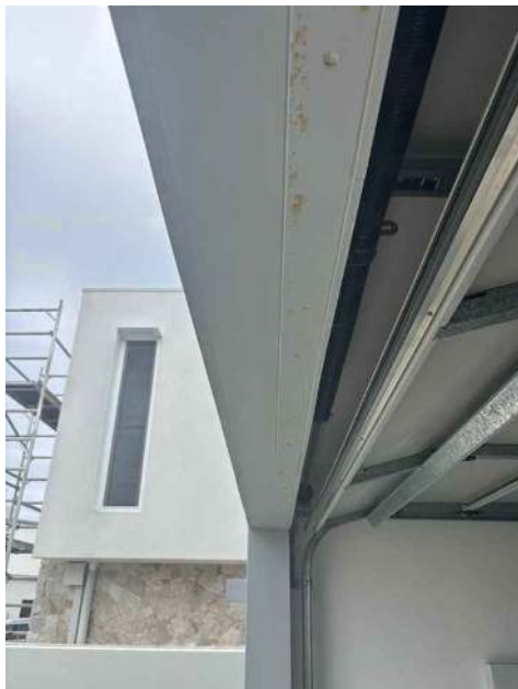
Eave / fascia and downpipe at an upper level with rust-coloured staining around the fixings — early-corrosion indicator at a downpipe bracket location (Items 19–20).
