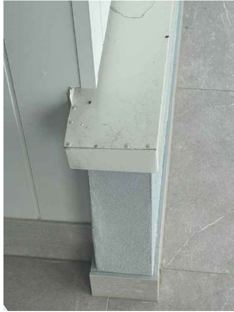
Upper flashing between 1st and ground floors - has been laid with a fall INTO the property.
