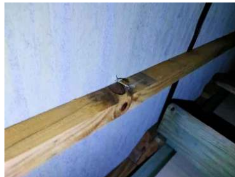
Roof-space view of a timber member with a metal bracket / bolt fixing against the membrane — fixing penetrations have missed battens.
