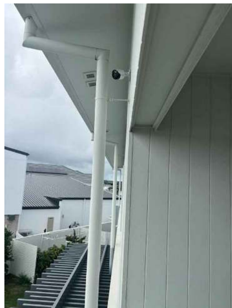
Downpipe and upper bracket at the eave / fascia running down past the cladding — upper bracket location relevant to the corrosion complaint (Items 19–20).
