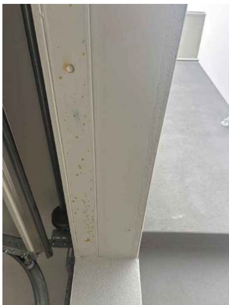
Interior structural post / column with bolt fixings and rust-coloured spotting — exposed steel showing early-corrosion indicators (Items 1–7).
