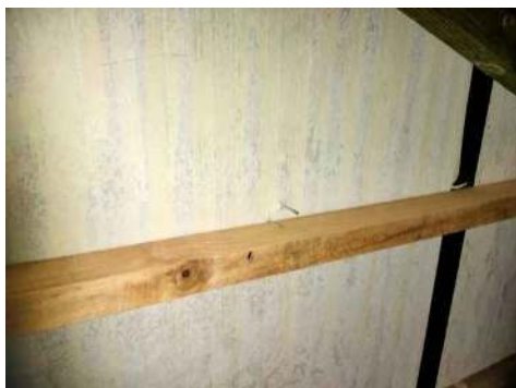
Roof-space view of timber framing against the wall lining fixings missing battens
