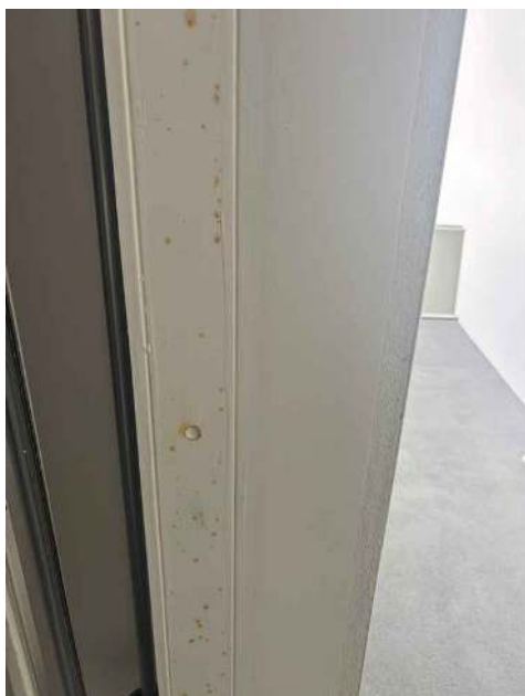
Interior wall / column junction with rust-coloured staining and spotting — coating breakdown / early corrosion at a structural interface (Items 1–7).
