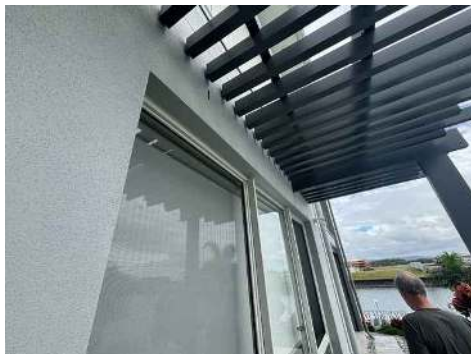
Downpipe fixed to the Axon-clad wall — upper bracket location relevant to the corrosion complaint (Items 19-20).
