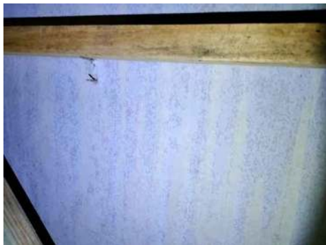
Roof-space view of a steel/timber member with rust-coloured staining against the sarking behind the cladding — early-corrosion indicator relevant to the durability assessment.
