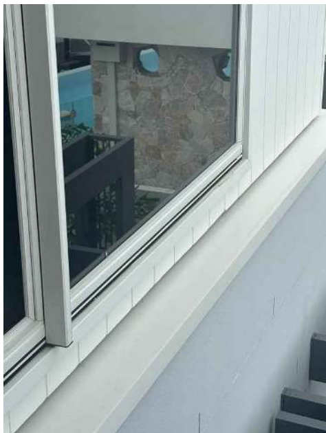
Upper-level window corner with insect screen — outdoor / canal area reflected; window perimeter detailing relevant to the flashing assessment (Items 13–18).
