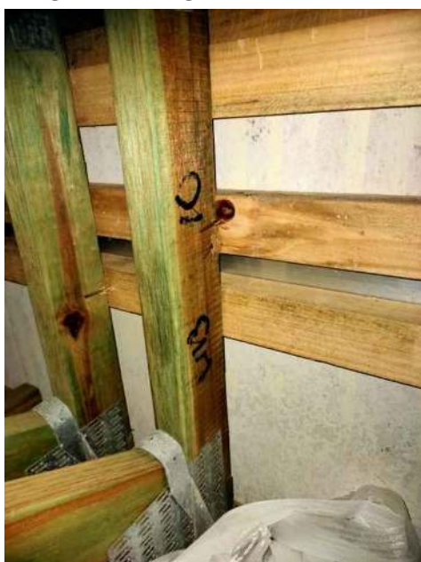
Roof-space view of timber framing against the wall lining fixings missing battens
