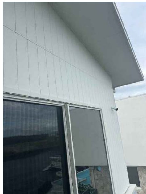
Upper-level gable windows in raking Axon cladding with the eave at the apex and canal beyond — head-flashing condition in dispute (Items 13–18).
