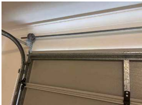
Garage opening head / lintel zone viewed from within the garage (sectional door and head) — corresponding to the garage lintel reported as unmarked and significantly corroded (Item 3).
