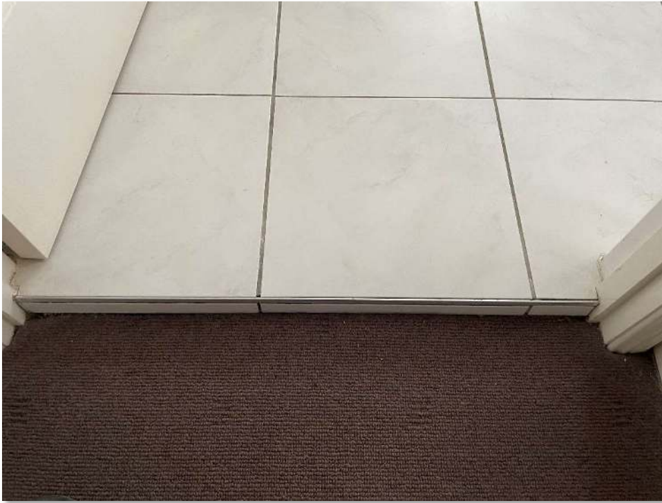
PHOTOGRAPH 1. NO WATER STOP TO BATHROOM ENTRY
