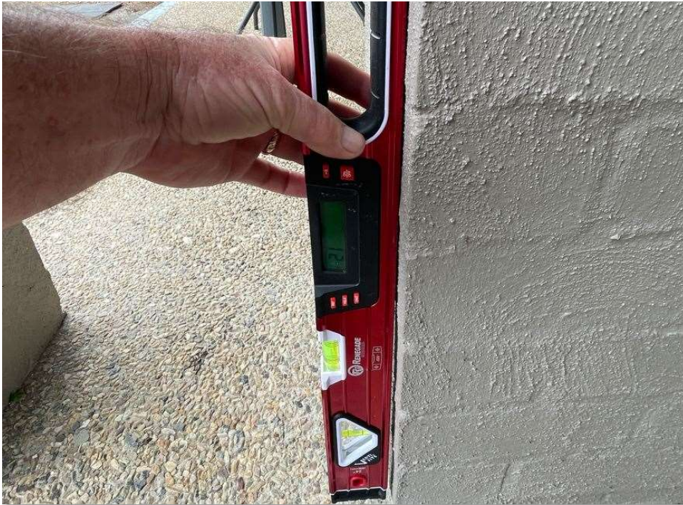
PHOTOGRAPH 3. BRICK PIER 21MM/MTR OUT OF PLUMB
