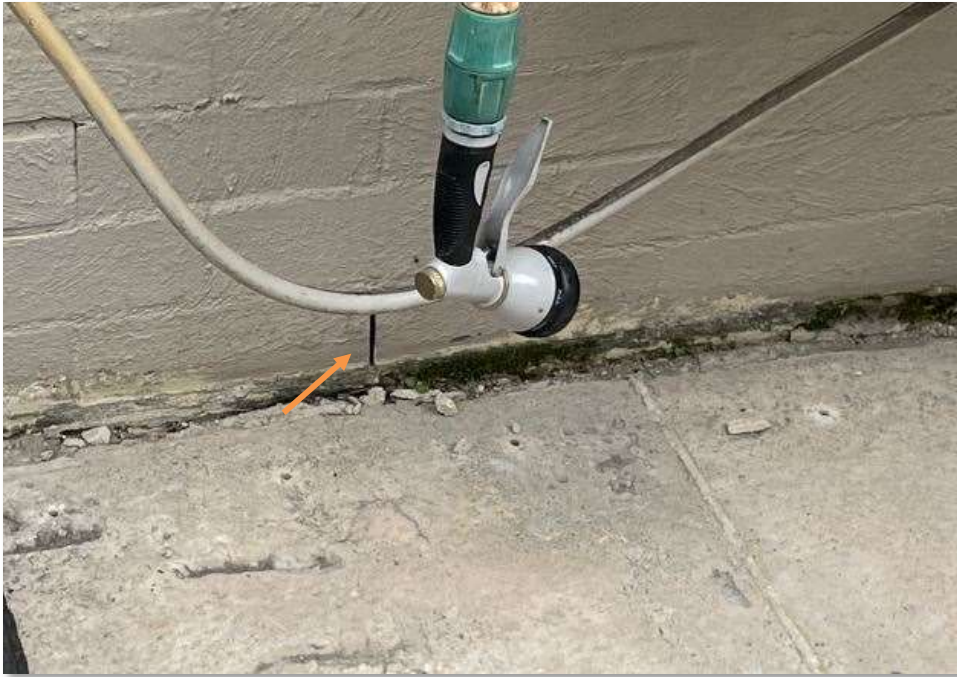
PHOTOGRAPH 9. LOW CLEARANCE ON WEEP HOLES
