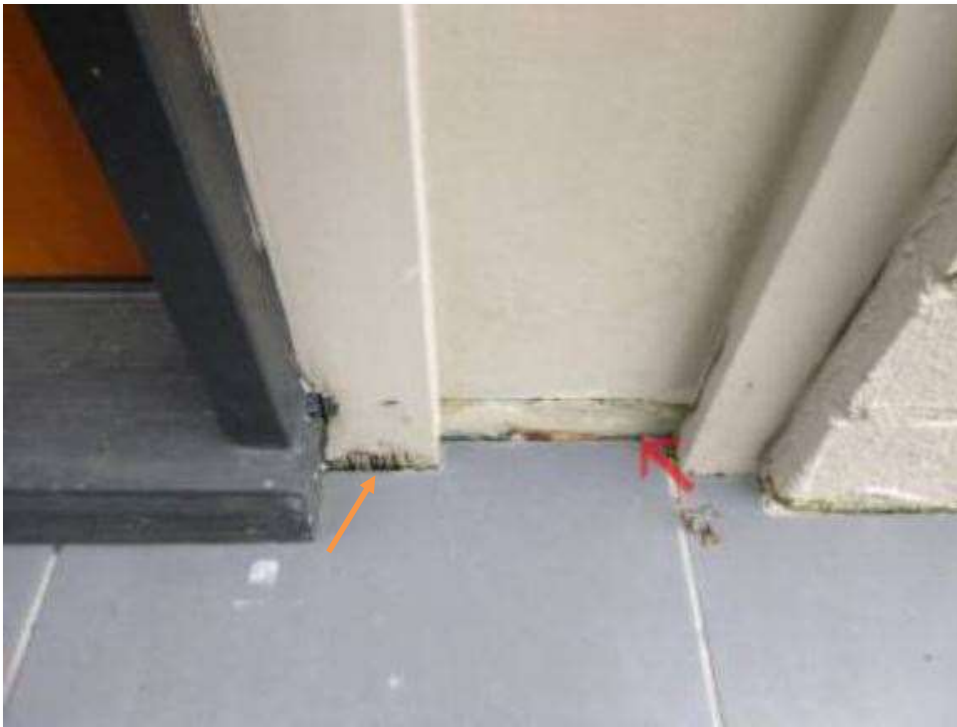
PHOTOGRAPH 10. NO GROUND CLEARANCE FOR TERMITE INSPECTION
