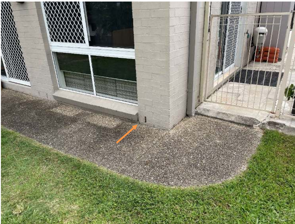
PHOTOGRAPH 8. LOW CLEARANCE ON WEEP HOLES
