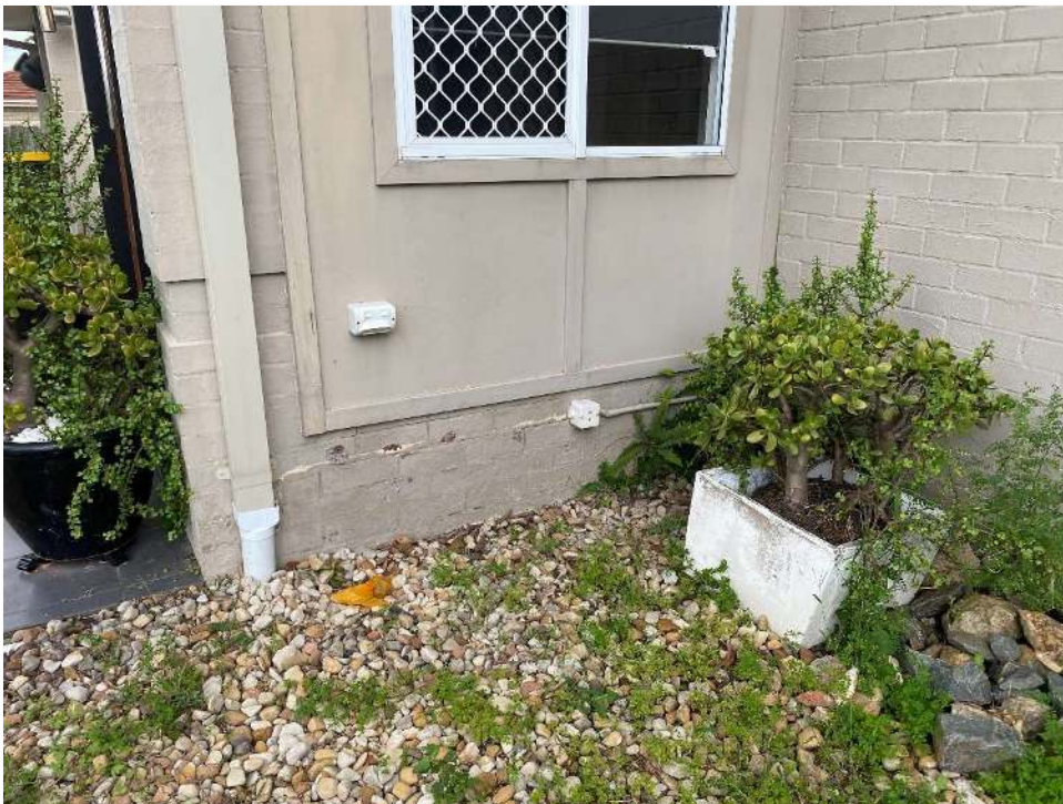
PHOTOGRAPH 6. NO DAMP COURSE
