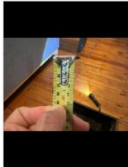
50mm W Joists
