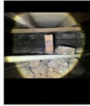
Section of the timber that are not supported Not structural Element
