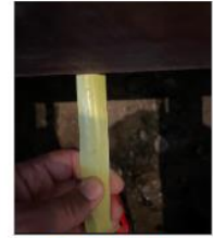
50mm W Joists
